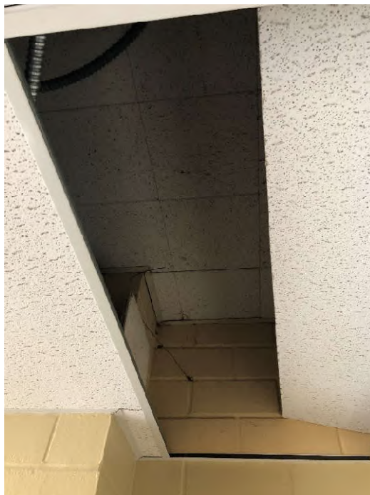
PHOTO 8: Shows the 1'x1', ceiling tile with crater pattern sampled above the ceiling grid located in the north foyer (Samples CT-04-26 through CT-04-28). Testing of this material did not indicate the presence of asbestos.
