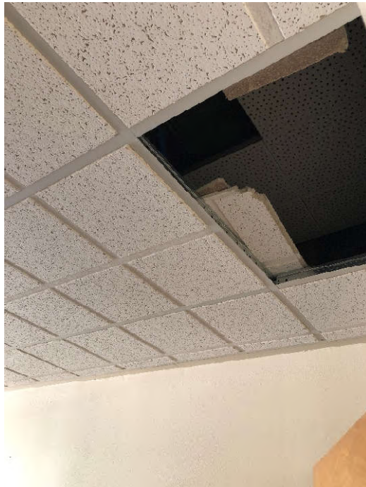
PHOTO 6: Shows the 2'x4', ceiling tile with 1'x1' inset pattern sampled in the office located across from the center storage room (Samples CT-02-20 through CT-02-22). Testing of this material did not indicate the presence of asbestos.
