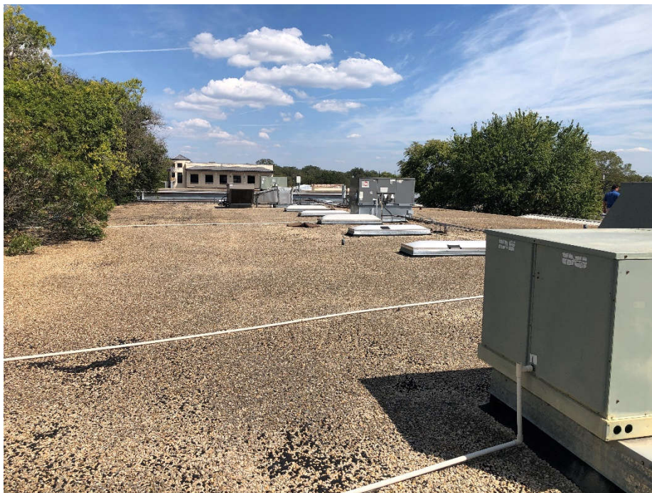
PHOTO 20: Shows the flat, gravel and tar roof of the building (Samples RC-01-62 through RC-01-64). Testing of this material did not indicate the presence of asbestos.
