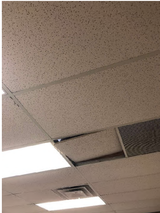
PHOTO 10: Shows the 2'x4', ceiling tile with pinhole and crater pattern sampled in the Business Office area (Samples CT-05-32 through CT-05-34). Testing of this material did not indicate the presence of asbestos.
