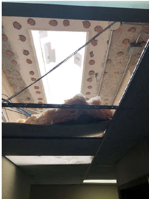
PHOTO 4: Shows the brown mastic sampled from the concrete ceiling deck in the common hallway (Samples CM-01-14 through CM-01-16). Testing of this material did not indicate the presence of asbestos.
