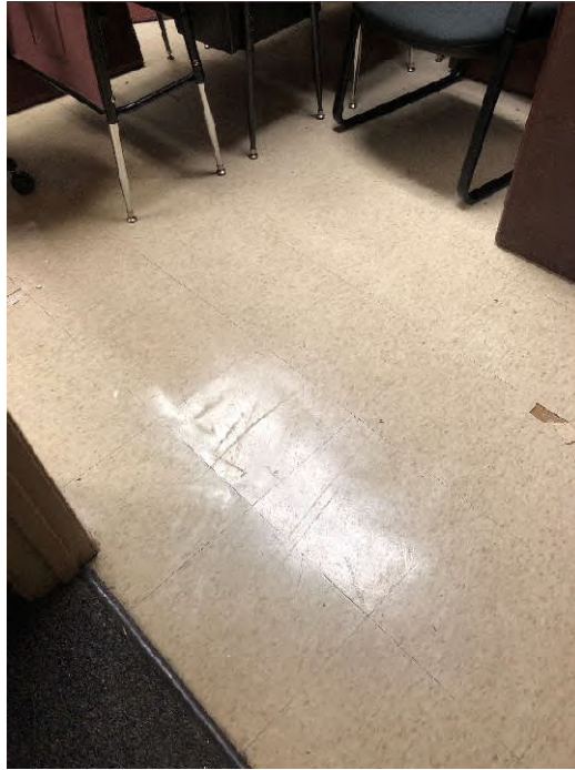
PHOTO 13: Shows the beige, 12”x12”, vinyl floor tile with tan splotches and yellow mastic sampled in the Dining Room (Samples VCT-02-41 through VCT-02-43). Testing of this material did not indicate the presence of asbestos.
