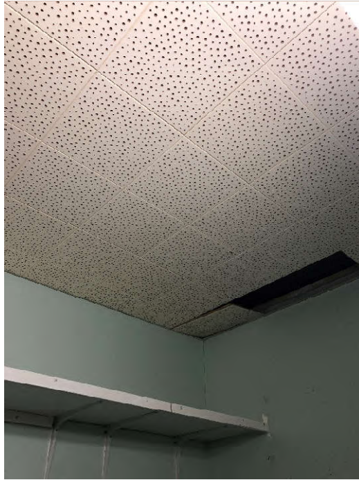
PHOTO 7: Shows the 1'x2', ceiling tile with pegboard pattern sampled in the center storage room (Samples CT-03-23 through CT-03-25). Testing of this material did not indicate the presence of asbestos.
