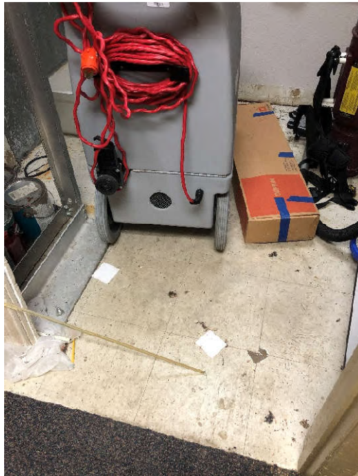
PHOTO 12: Shows the off-white, 12”x12”, vinyl floor tile with gray splotches and yellow mastic sampled in the Custodial Closet (Samples VCT-01-38 through VCT-01-40). Testing of this material did not indicate the presence of asbestos.
