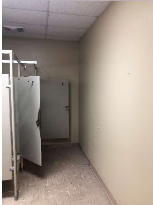
PHOTO 15: Shows the tan, 12"x12", vinyl floor tile with beige and brown streaks and yellow mastic sampled in the main men's and women's restrooms (Samples VCT-04-47 through VCT-04-49). Testing of this material did not indicate the presence of asbestos.
