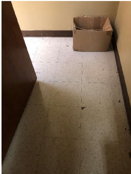
PHOTO 14: Shows the white, 12”x12”, vinyl floor tile with blue and gray splotches and yellow mastic sampled in the Board Room Restroom (Samples VCT-03-44 through VCT-03-46). Testing of this material did not indicate the presence of asbestos.
