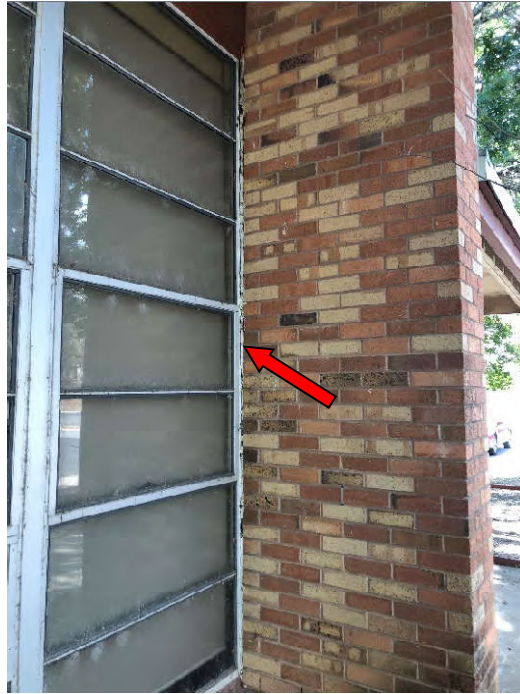
PHOTO 23: The red arrow indicates the window caulking sampled in between the metal window frame and the brick veneer (Samples WC-01-71 through WC-01-73). The caulking indicated the presence of asbestos at a concentration of two (2) percent.
