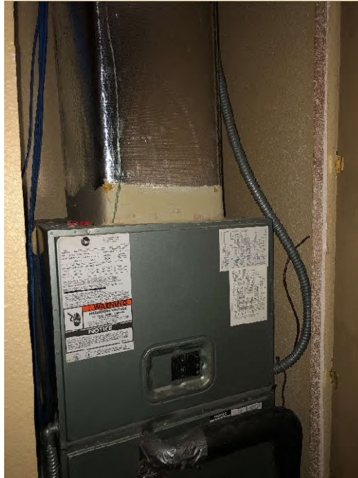
PHOTO 9: Shows the off-white mastic on HVAC duct sampled in the HVAC closet located in the IT Server Room (Samples HVAC-01-29 through HVAC-01-31). Testing of this material did not indicate the presence of asbestos.
