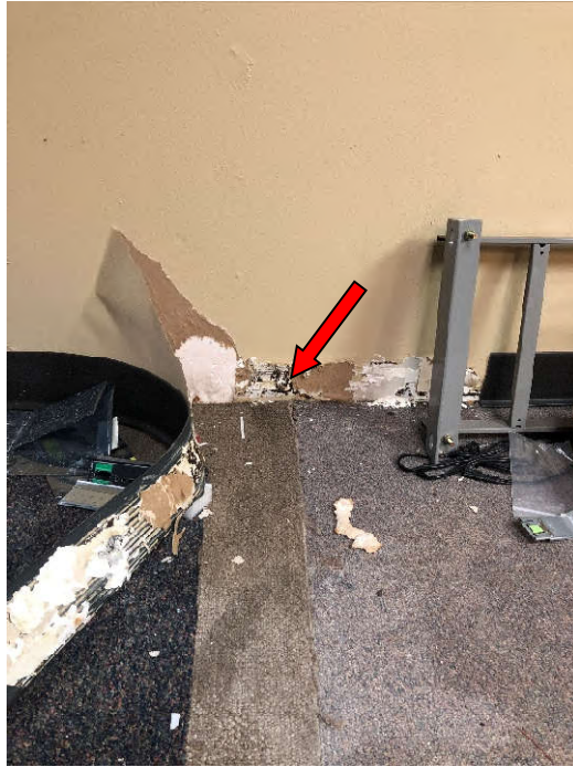
PHOTO 11: Shows the brown baseboard mastic sampled in the IT Server Room (Samples WM-01-35 through WM-01-37). Testing of this material did not indicate the presence of asbestos.
