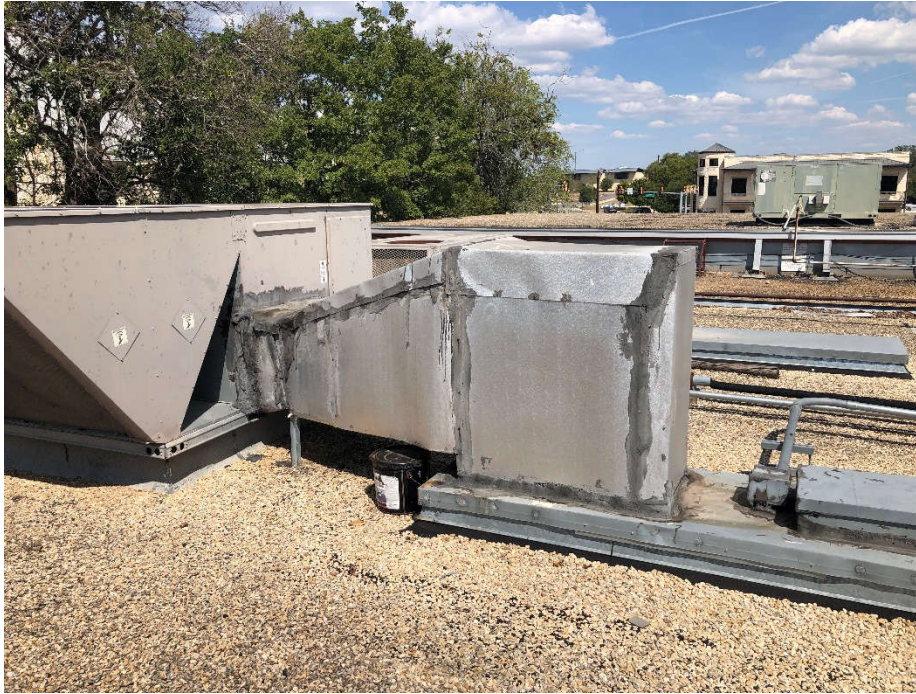
PHOTO 21: Shows the black/gray mastic sampled from metal HVAC duct located on the roof of the building (Samples HVAC-02-65 through HVAC-02-67). Testing of this material did not indicate the presence of asbestos.
