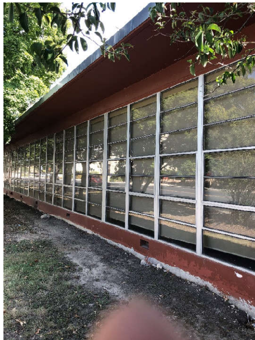
PHOTO 22: Shows the windows located on the north side of the building where residual window glazing was sampled (Samples WG-01-68 through WG-01-70). The residual window glazing indicated the presence of asbestos at a concentration of two (2) percent.
