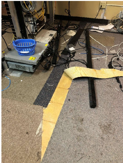
PHOTO 18: Shows the beige, 9"x9", vinyl floor tile with black mastic sampled in the IT Server Room (Samples VCT-07-56 through VCT-07-58). The black mastic and vinyl floor tile indicated the presence of asbestos at a concentration of two (2) percent.
